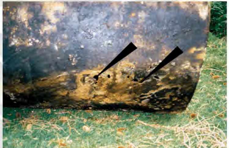
(Above) Example of a typical UST with large pin-hole perforations
